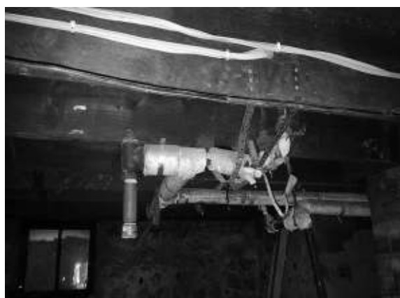
Photo #5: View of TSI pipe wrap on horizontal pipe chase in basement (September 5, 2017)
