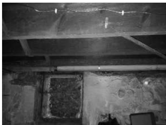
Photo #4: View of TSI pipe wrap on horizontal pipe chase in basement (September 5, 2017)
