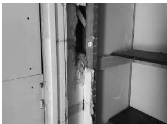
Photo #3: View of plaster and insulation in interior of the house (September 5, 2017)
