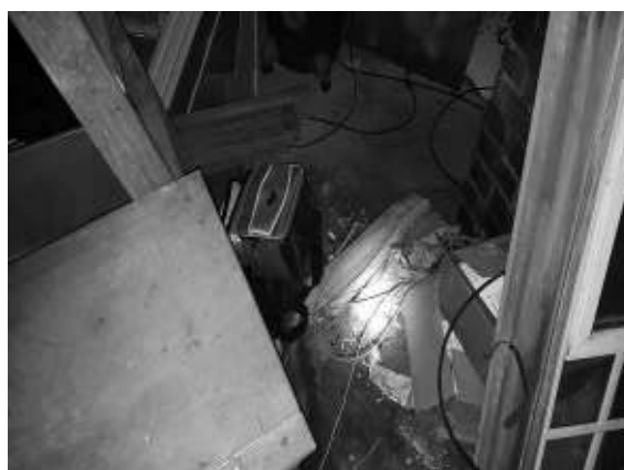
Photo #6: View of damaged TSI pipe wrap on floor in basement (September 5, 2017)
